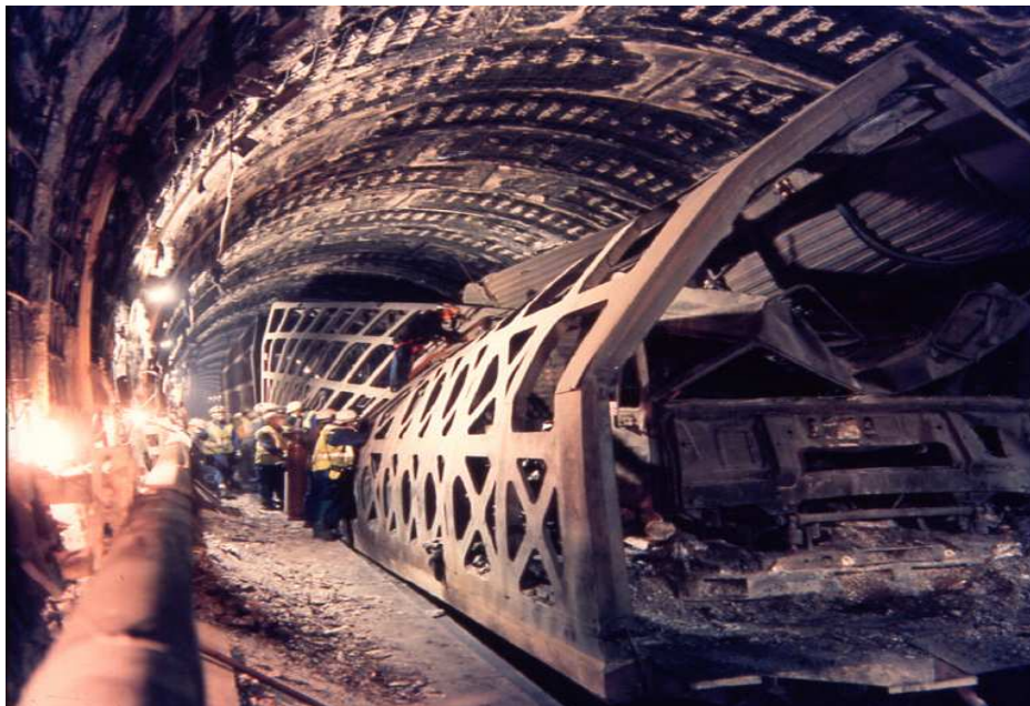
Fig. 1 Damage in the channel tunnel 1996
