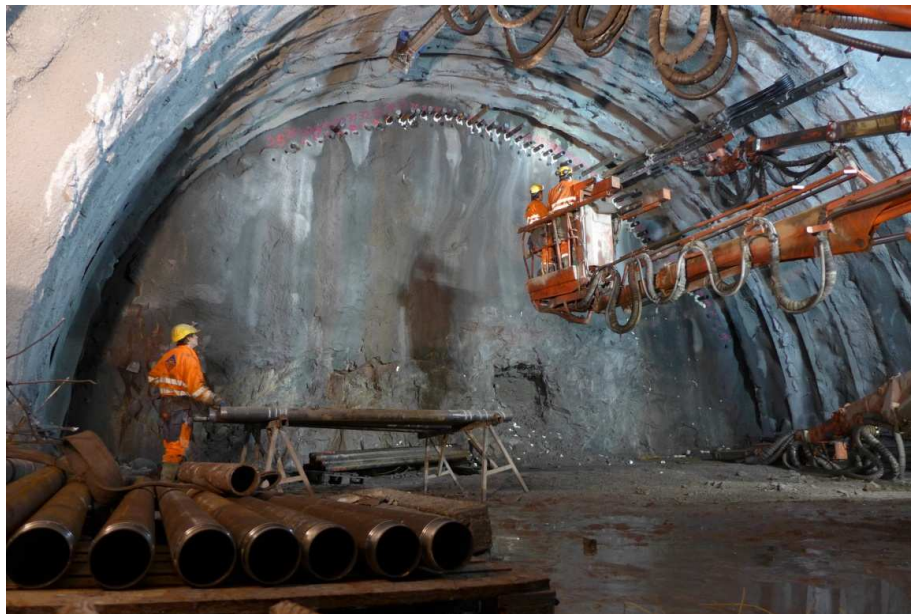
Obr. 4 Vrtanie dáždnika v tuneli Fegstad Fig. 4 Drilling the canopy tube pre-support in the Fegstad tunnel
