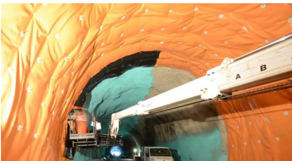
Obr. 2 Realizácia hydroizolácie v bezpečnostnom tuneli Mitholz oboma technikami Fig. 2 Waterproofing realization in the safety tunnel Mitholz with both techniques
