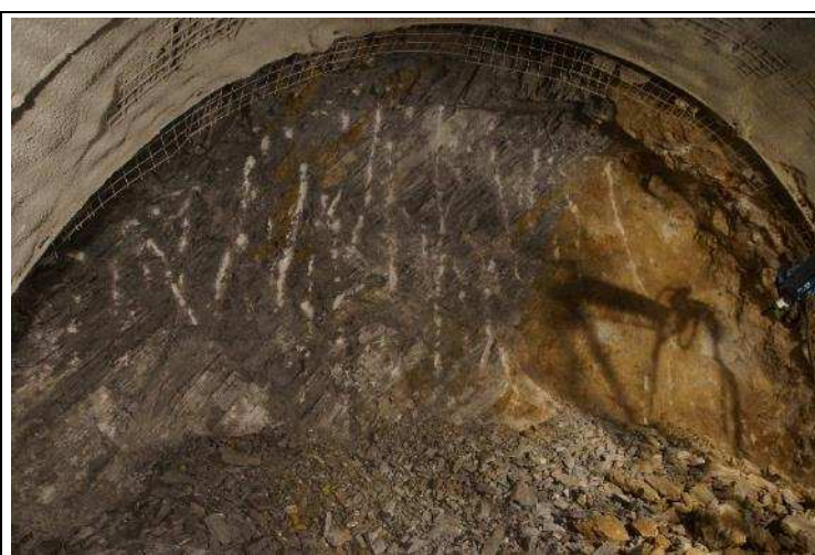
Obr. 19 Sklony diskontinuit na čelbě Fig. 19 Dipping of discontinuities at the excavation face
