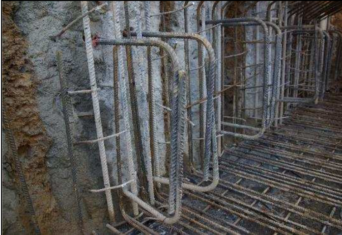
Obr. 4 Obnažená výztuž pilot a vlepená kotevní železa pro napojení želvy Fig. 4 Exposed reinforcement of piles and the anchoring steel fixtures glued into them for connecting the “tortoise shell” structures to them
