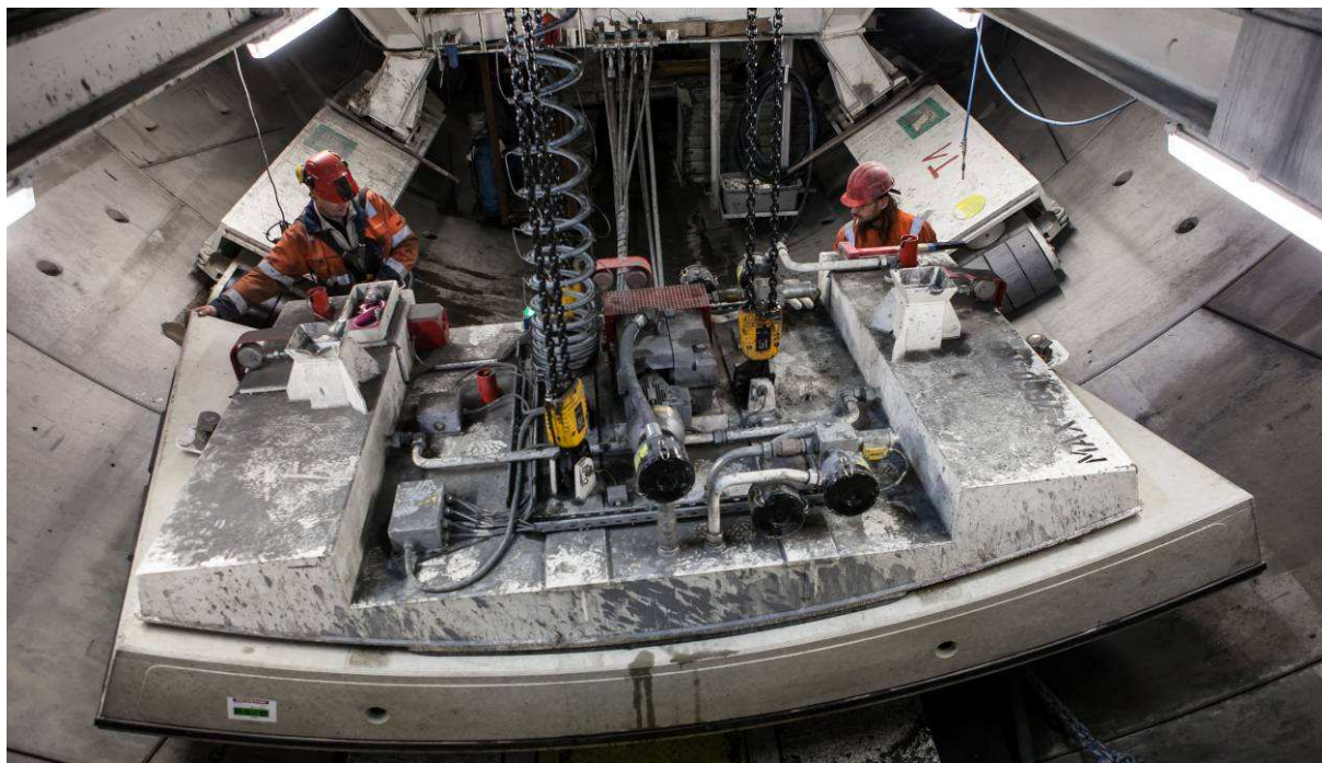
Obr. 8 Manipulácia s tybinkami v útrobách tunelovacieho stroja Fig. 8 Manipulation with the segment inside the tunneling machine
