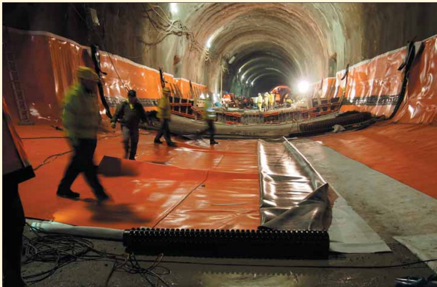
Obr. 4 Tunel Mezno, betonáž sekundárního ostění v profilu s protiklebou Fig. 4 Mezno tunnel, concreting of the secondary lining in the profile with the invert
