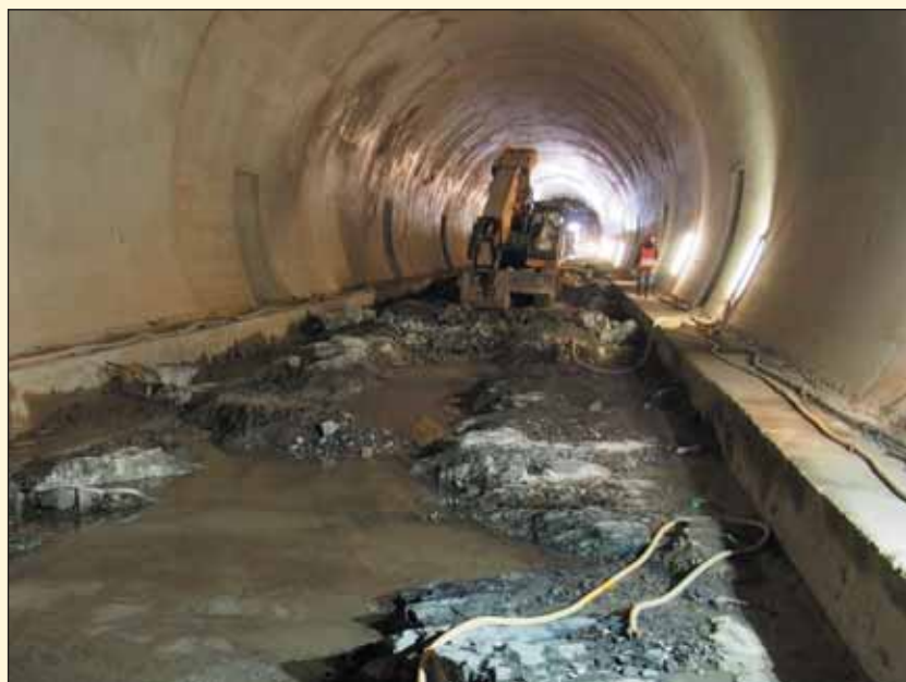
Obr. 5 Tunel Deboreč, čištění a betonáž dna tunelu Fig. 5 Deboreč tunnel, cleaning and concreting of the tunnel bottom
