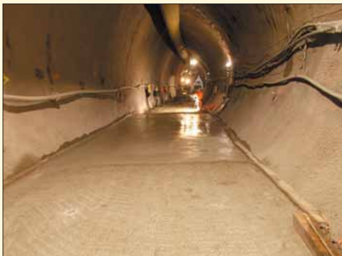
Obr. 2 Lokalita VO-OL, pohled na vyraženou štolu Fig. 2 Locality VO-OL, a view down the excavated gallery
