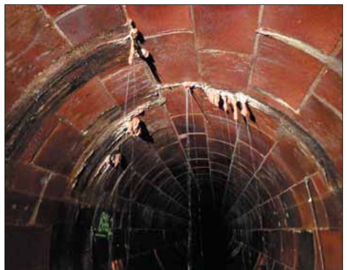
Obr. 7 Infiltrace vody z rubu obezdívky do stoky Fig. 7 Water infiltration from the sewer extrados
