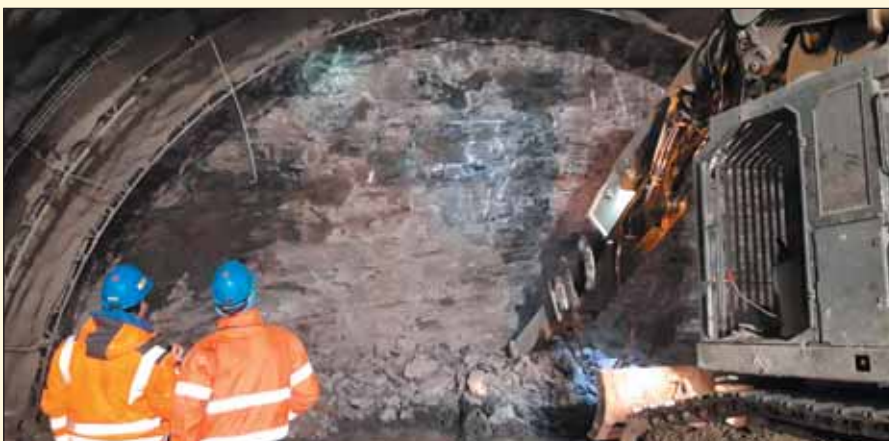
Obr. 3 Čelba kaloty tunelu Mezno v TM 348 Fig. 3 Mezno tunnel excavation face at tunnel chainage m 348
