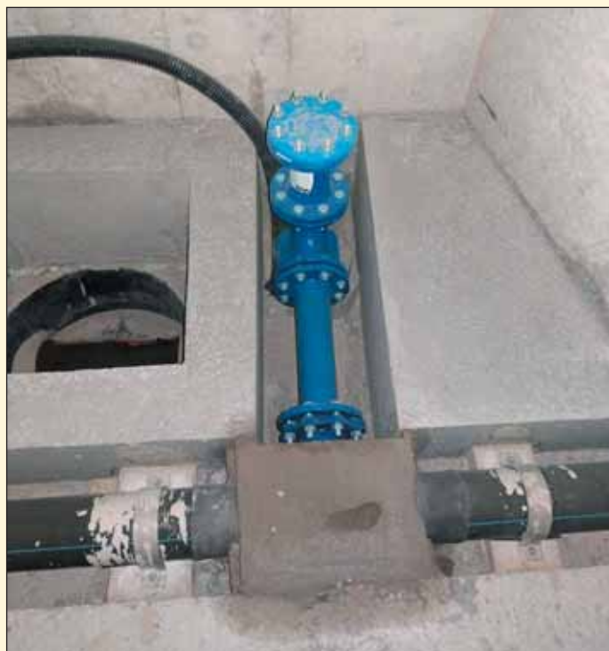
Obr. 5 Suchovod tunelu Diel Fig. 5 Dry fire main in the Diel tunnel
