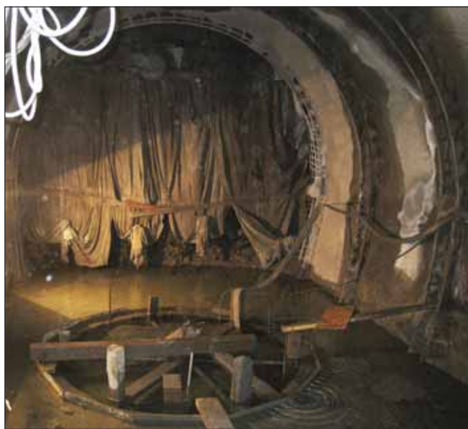
Obr. 9 Pohled do komory s ohlubní šachty Fig. 9 View down the chamber with the shaft pit completed
