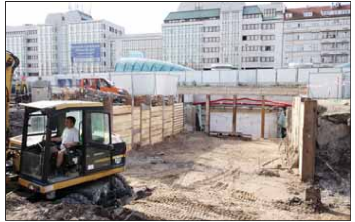
Obr. 8 Na Hradčanské probíhá dostavba podchodu pod tratí ČD směrem do Dejvic Fig. 8 Completing of the pedestrian subway under Czech Railways track toward Dejvice is underway at Hradčanská metro station
