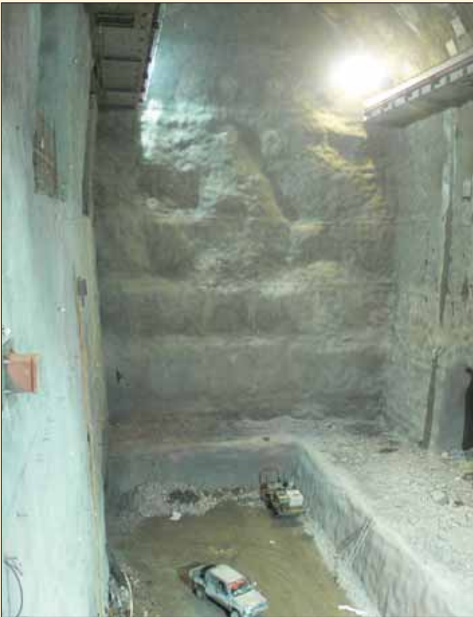
Obr. 2 Pohled do kaverny strojovny PVE Fig. 2 View of the cavern of the pumped storage power station machine room
