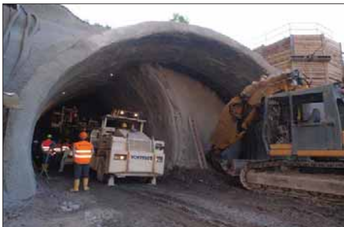
Obr. 5 Ražba dvojkolejného tunelu ze stanice Motol (foto J. Junek) Fig. 5 Driving the double-track tunnel from Motol station (photo courtesy of J. Junek)
