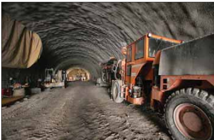
Obr. 1 Dvojkolejný tunel za stanicí Motol (foto J. Husák) Fig. 1 Double-track tunnel behind Motol station (photo courtesy of J. Husák)
