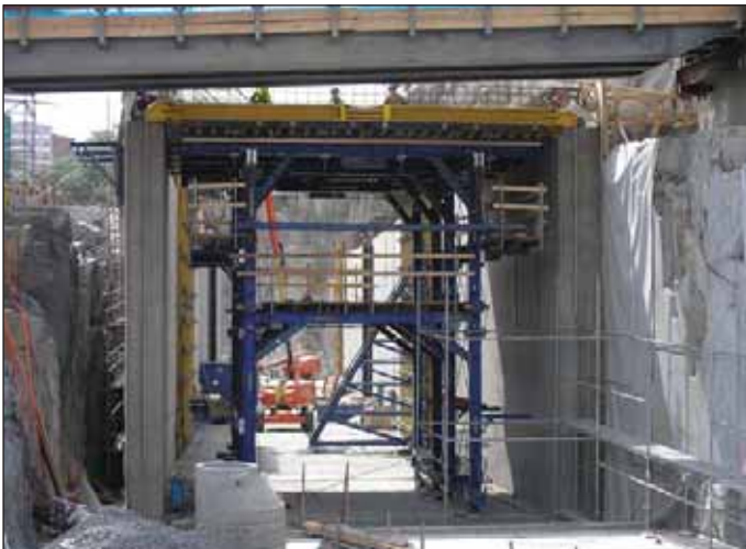
Obr. 8 Debniaci voz na stropnú dosku tunela I12 Fig. 8 Travelling formwork for the roof deck of tunnel I12
