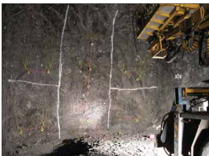
Obr. 5 Nabíť a zapojená čelba tunela III Fig. 5 Charged and wired face of tunnel III
