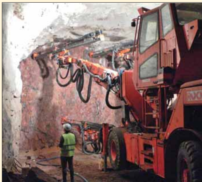
Obr. 3 Pohled na čelbu tunelu raženého v charakteristicky zbarvené finské žule Fig. 3 View of the excavation face of the tunnel driven through the characteristically coloured Finnish granite
