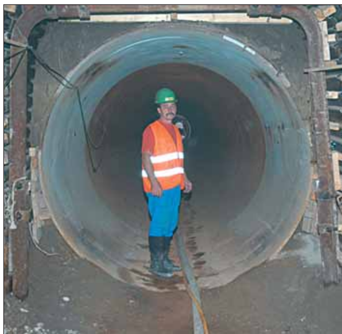
Obr. 3 Rozhraní protlaku a klasické štoly Fig. 3 The interface between the pipe jack and traditional tunnel
