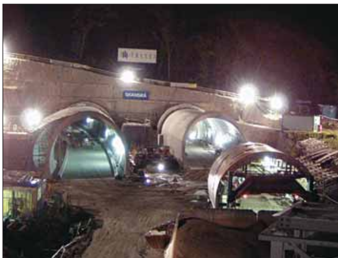
Obr. 8 Stavebné práce na južnom portáli tunela Sitina Fig. 8 Construction work on the south portal of the Sitina tunnel
