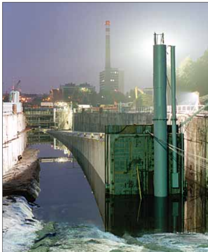
Obr. 22 Vysouvané tunely pod Vltavou na prodloužení trasy „C“ metra Fig. 22 Immersed tunnels of the Line “C” extension crossing the Vltava River before launching
