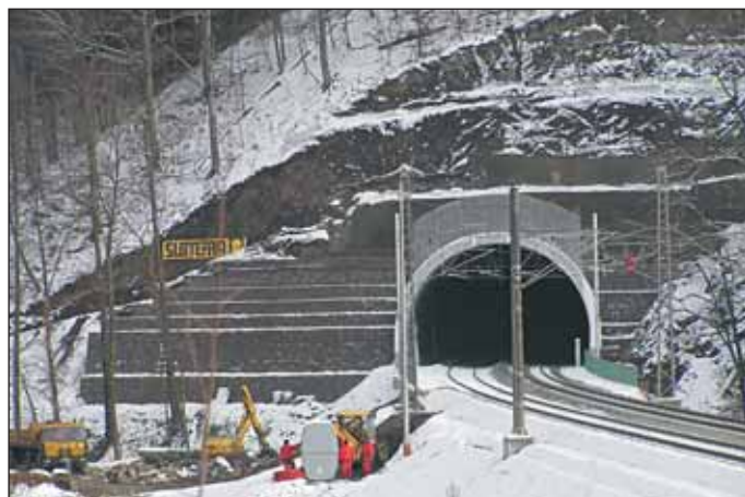
Obr. 4 Tunel Malá Huba – vjezdový portál Fig. 4 The Malá Huba Tunnel entrance portal
