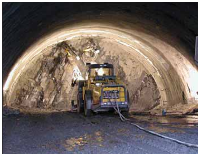
Obr. 3 Čelba kaloty tunelu Klimkovice Fig. 3 The Klimkovice tunnel – the top heading face
