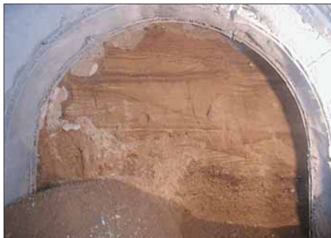
Obr. 26 Kolektor Vodičkova v Praze v průběhu ražby Fig. 26 The utility tunnel under Vodičkova Street in Prague during the course of the excavation
