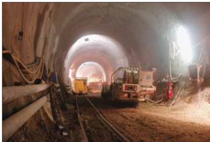
Obr. 6 Kolajová technológia odťahby s nakladačom Fig. 6 Track-bound mucking out equipment with a loader
