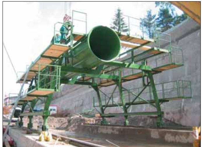
Obr. 4 Montáž plošiny na staveništi Fig. 4 Installation of the platform at construction site
