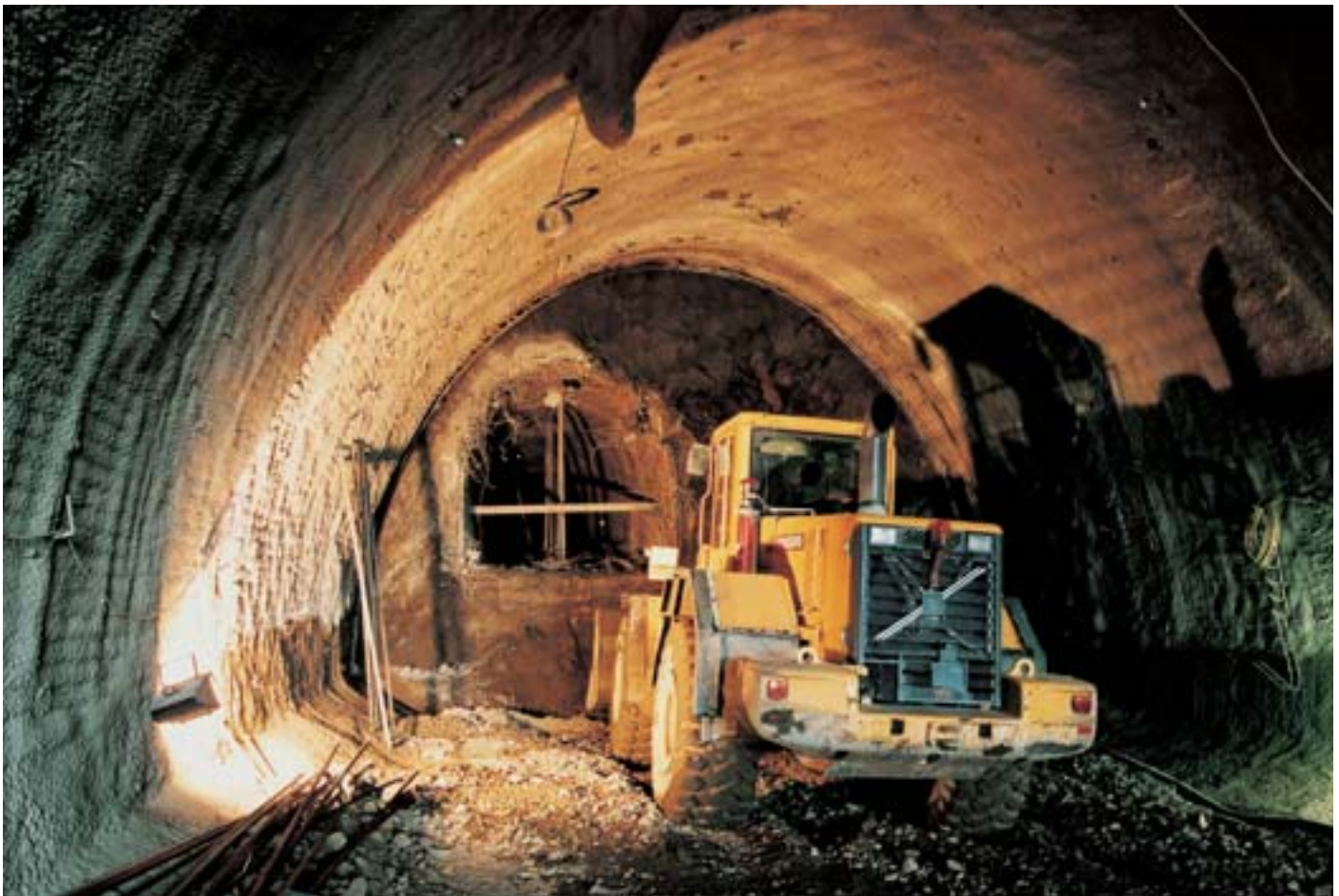
Obr. 3 Tunel Valík – čelba stredného tunelu Fig. 3 Valík Tunnel – from of the middle tube
